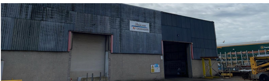
Last year, AJE embarked on a project to replace the rails, purlins, roof and wall cladding on Highland Galvanisers Elgin building
